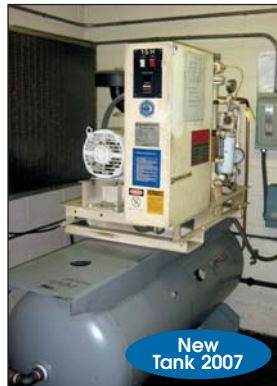
INGERSOLL-RAND 15 HP AIR COMPRESSOR
