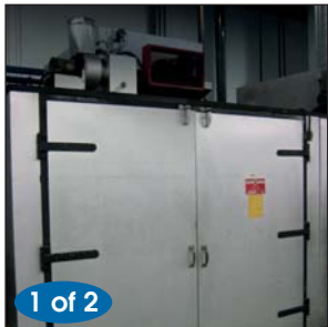
GEHRICH BATCH OVENS
