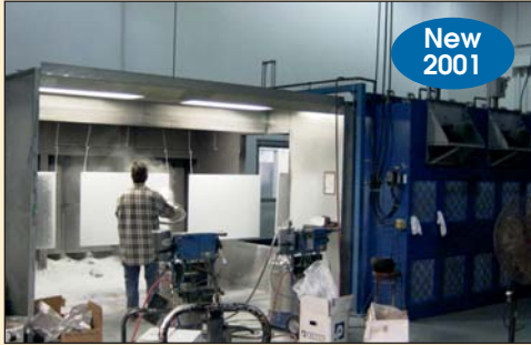
NORDSON POWDER COAT PAINT SYSTEM
