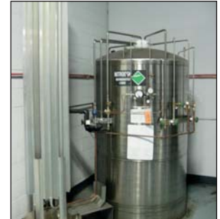
VIEW OF NITROGEN TANKS
