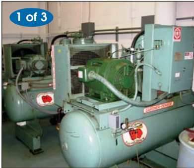
GARDNER-DENVER 30 HP AIR COMPRESSORS
