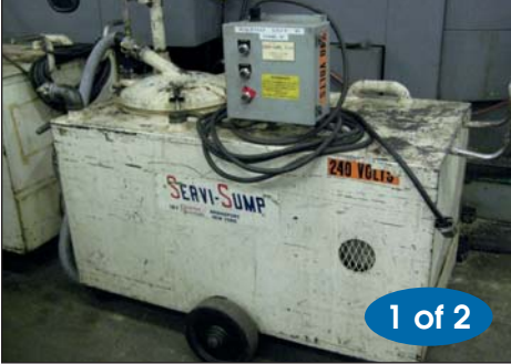
SERVI-SUMP OIL RECOVERY SYSTEM
