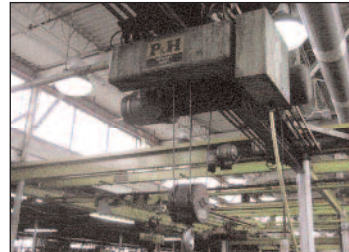
VIEW OF P&H 3 TON HOIST
