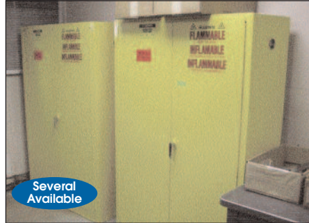
FLAMMABLE STORAGE CABINETS
