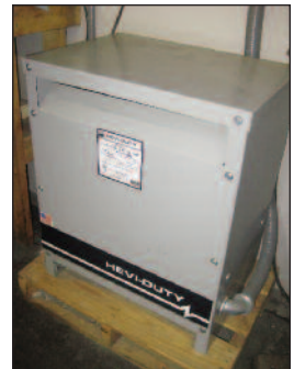
SEVERAL LARGE TRANSFORMERS
