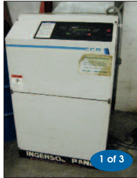
INGERSOLL-RAND 30 HP ROTARY SCREW AIR COMPRESSOR # SSP-EP30SE
