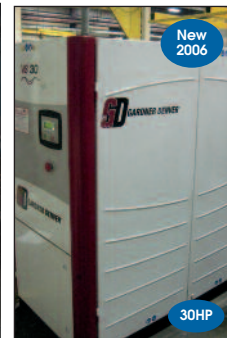
GARDNER DENVER # VS-30 ROTARY SCREW AIR COMPRESSOR
