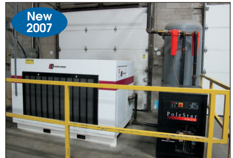
GARDNER DENVER EAM99C COMPRESSOR & DOMNICK HUNTER DRYER
